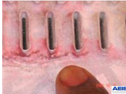
Figure7: Cracks in the header plate to tube joint of leaking radiator
