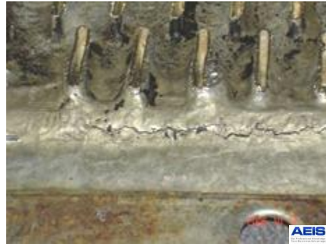
Figure 2: Crack along the edge of the cover plate of leaking radiator
