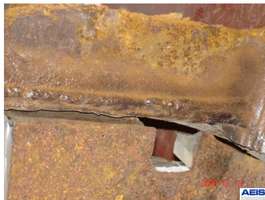
Figure 2: The main crack as viewed from inside the boom heel.
