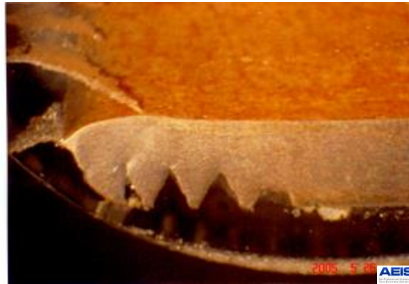
Figure 3: Evidence that fracture took place by a side load of the pipe
